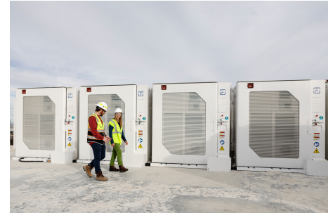
Once completed, 11.7 MW/34 MWh battery-based energy storage system co-located with a solar farm will produce enough energy to supply 5000 households with renewable, low-cost energy for an entire day.
